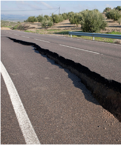
Seismically damaged road
