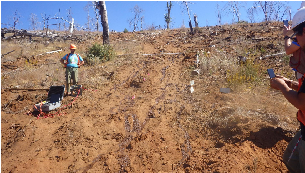
Standard water bar spacing prescribed by the California Forest Practice Rules (30 m): " Control "
