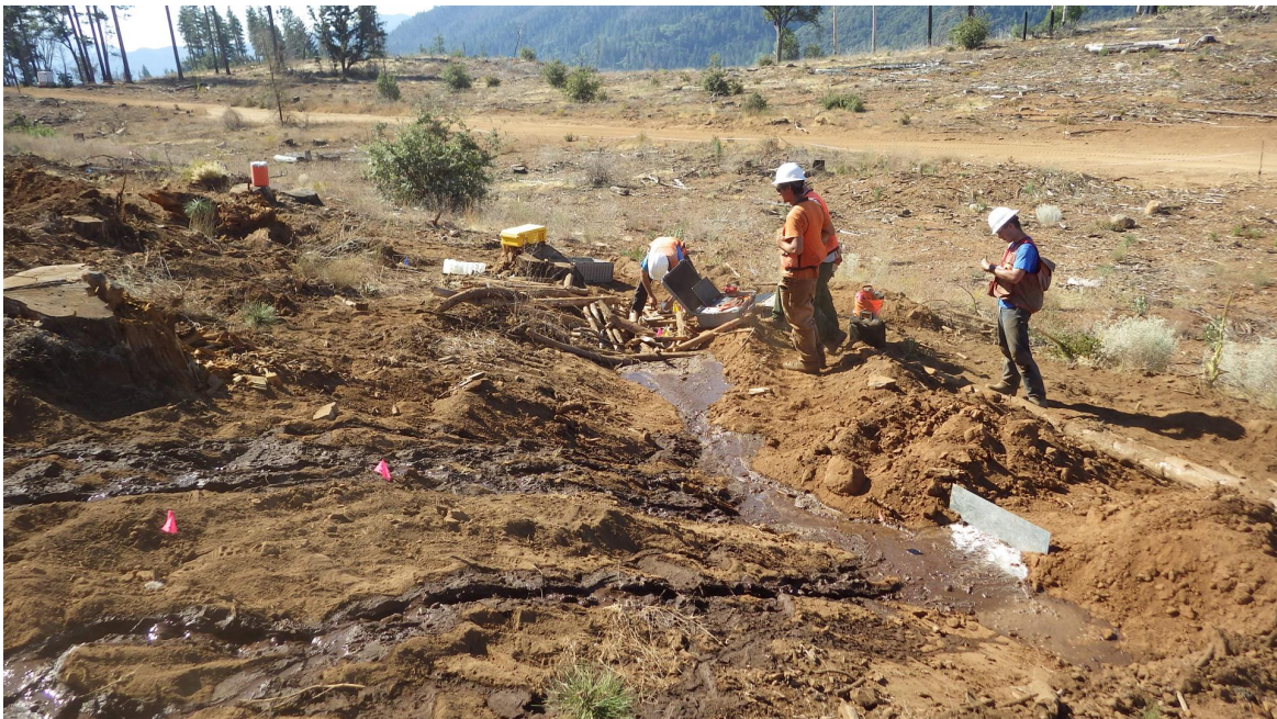
Water bar outlets covered with logging slash (70%), which was then driven over 2x with a heavy machine: " Slash-packed "
