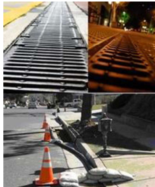
Figure 45: Storm Drain Debris Mitigation
