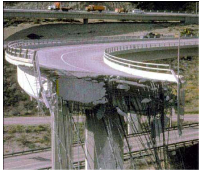
Figure 27: Freeway Collapsed Interchange
