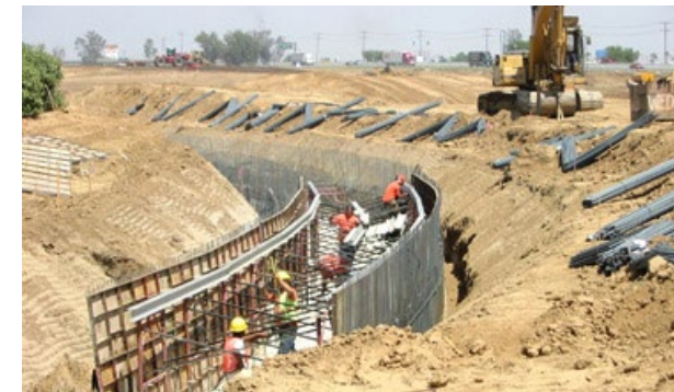
The RCFCWCD manages flood control projects such as the construction of the Nason Basin, above. In 2003, the District completed the construction of the 16-acre basin, which reduces the 100-year flows by more than 70%.
