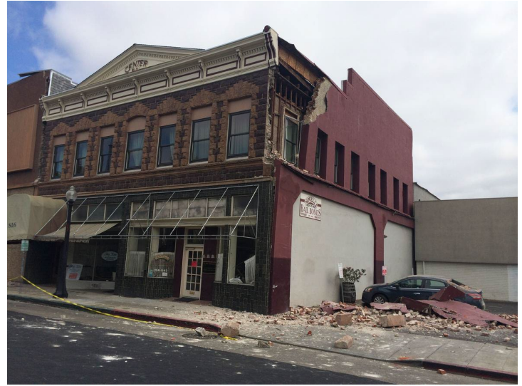
2014 South Napa Earthquake damaged unreinforced masonry building on Main St. in Napa Downtown. Courtesy of USGS
