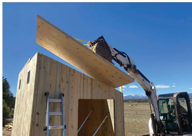
TimberAge Systems has scaled their CLT business to meet the needs of their rural community (photo courtesy of TimberAge Systems)
