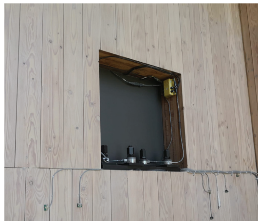
Moisture sensors at Oregon State University's Peavy Hall are used to detect moisture content of the mass timber panels
