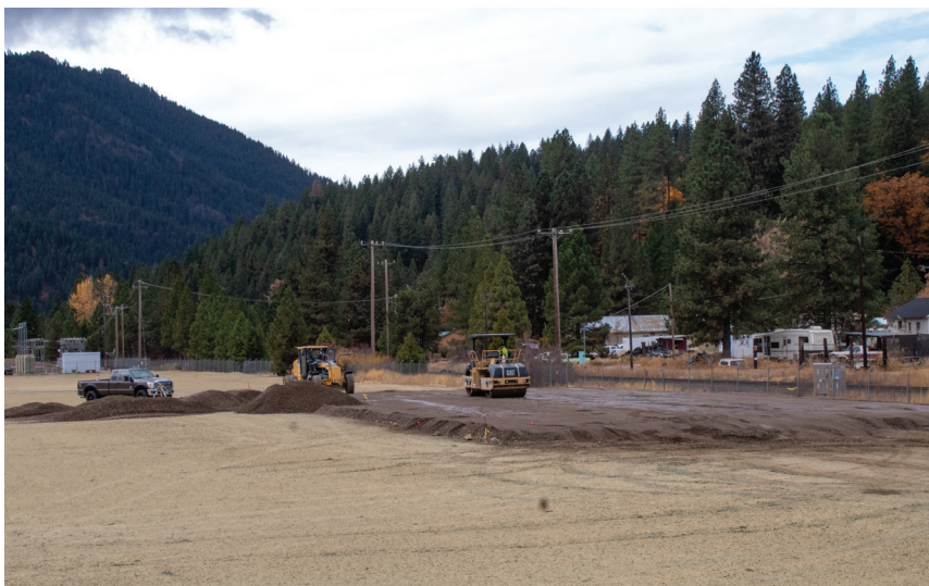
Brownfield remediation work to create a wood chips storage shed at Indian Valley Wood Products Campus in Crescent Mills, California
