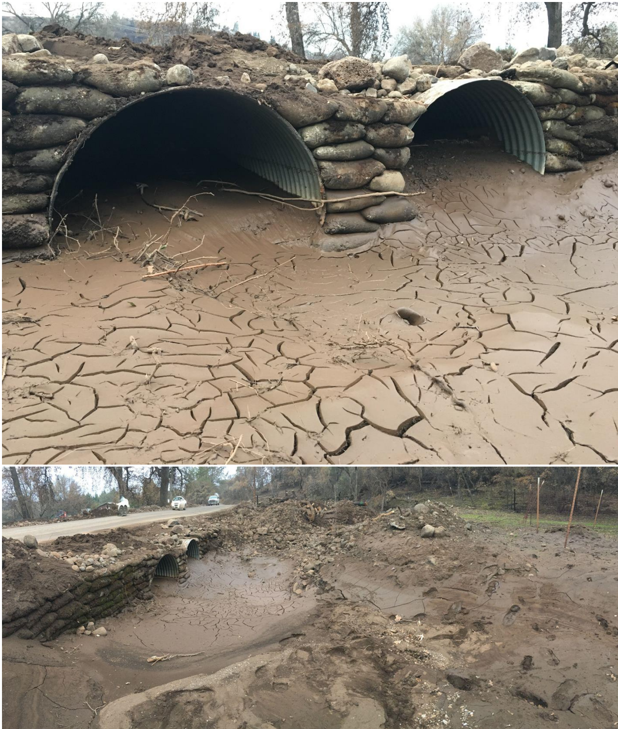
Figure 4-64 Butte County – Clogged Culverts after Erosion
