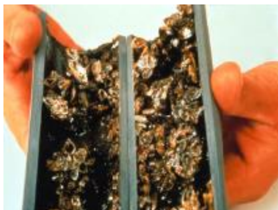
Figure 4-54 Mussels Clogging a Pipe
