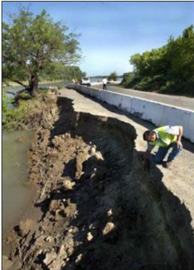
Figure 4-66 Erosion along River Road
