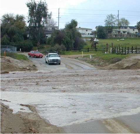
The 2010 storms flooded low water crossings and created safety hazards.
