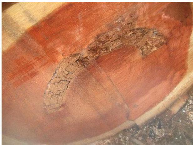
1948 Fire Damage – Defect Compartmentalized
