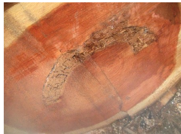
1948 Fire Damage – Defect Compartmentalized
