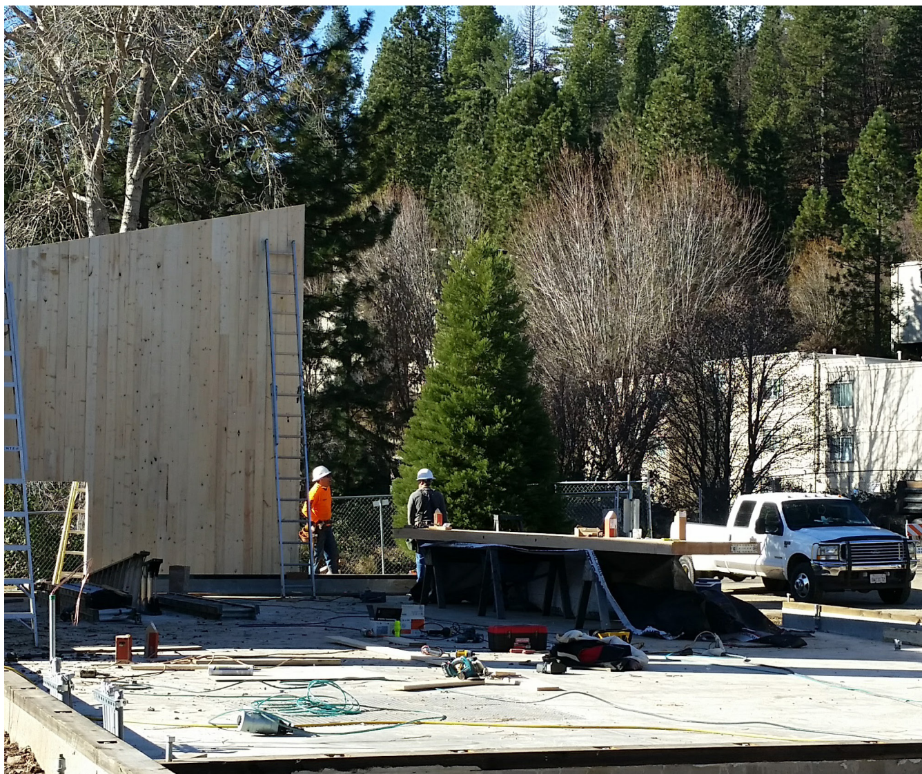
First cross laminated timber building in the State of California, under construction, Quincy, CA.
