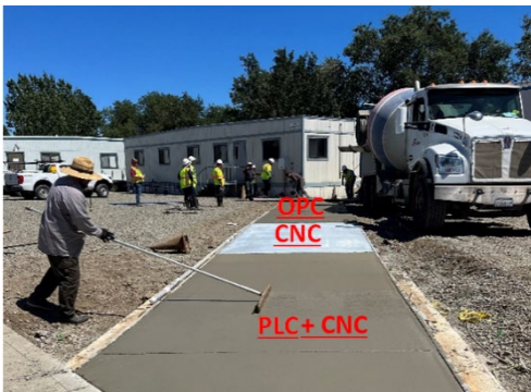
Figure 3. Field placement of mixtures 1) OPC (top slab in the picture) 2) OPC+CNC 3) PLC+CNC (bottom slab in the picture).
