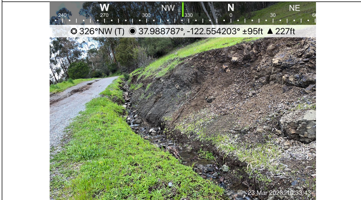
Photo 8. Wetted roadcut feature along fire road leading north from cemetery. (Reconnaissance Survey, 3/23/2023)
