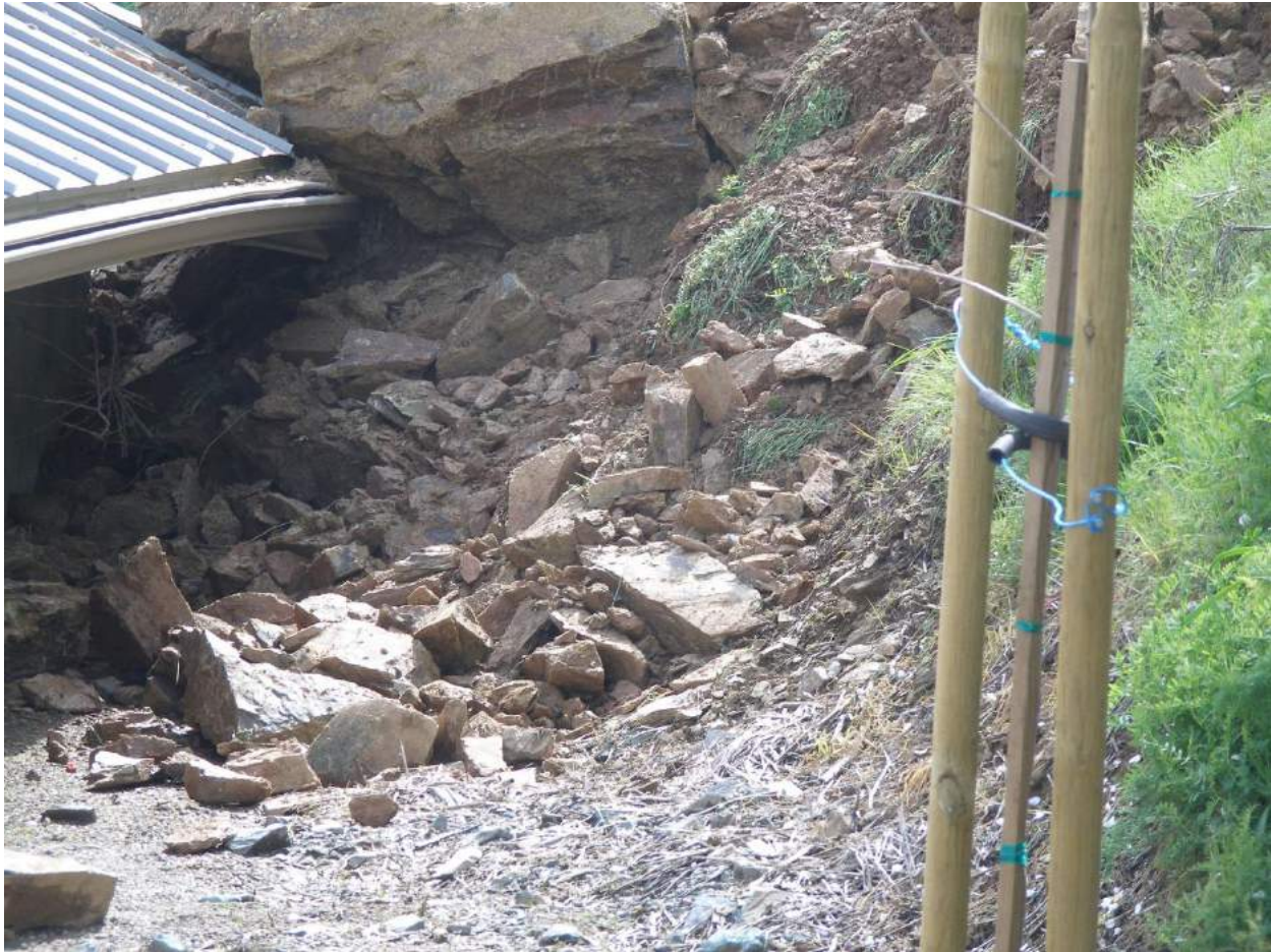
Figure C-14 City of Jackson – Past Damages from Landslide
