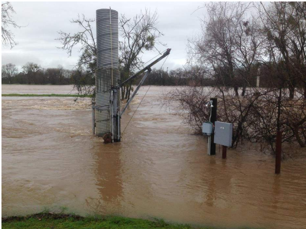
Figure I-7 Inundated Pumping Station 2017
