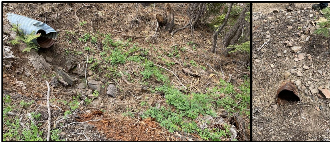
Figure 21: A Class III culvert crossing used for harvest operations that was not able to freely pass water and/or debris, and in need of maintenance and improvement.
