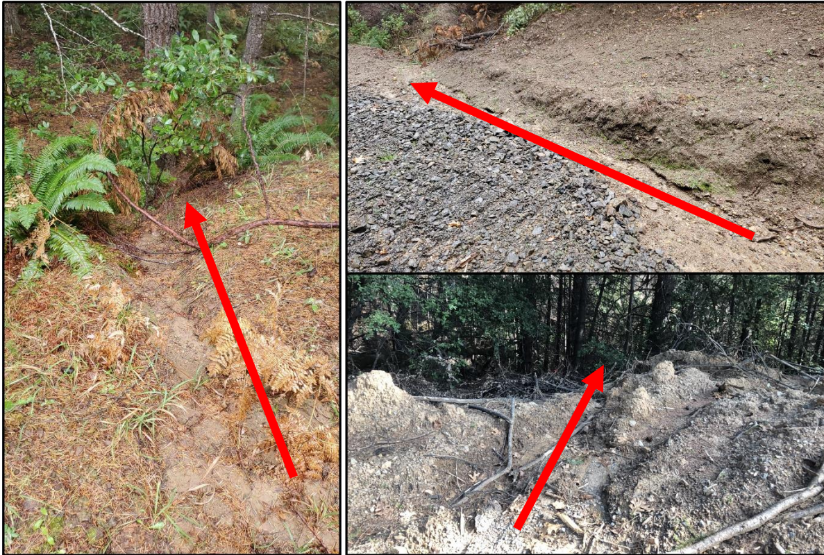
Figure 15: Road segment discharge points. Left, discharge below a waterbar into a Class III watercourse, top right a discharge point from a rolling dip onto bare soil into a Class III below, and bottom right sediment discharge below a road drainage point on bare soil with a Class III below. Red arrows indicate direction of runoff.
