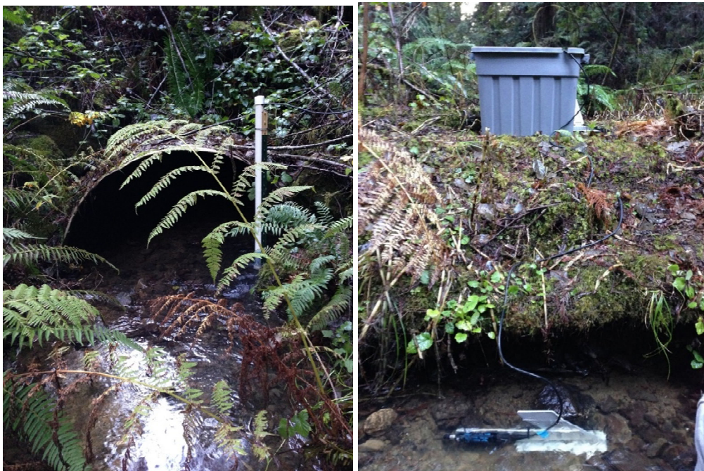
Figure 11. Left image: Standpipe for stage measurement at the inlet of the culvert on the Class I watercourse crossing; Blue Gum Creek JDSF road 600. Right image: Turbidity probe installed on the upstream side of the Class I watercourse crossing. The container on the bank contains the probe's data logger.
