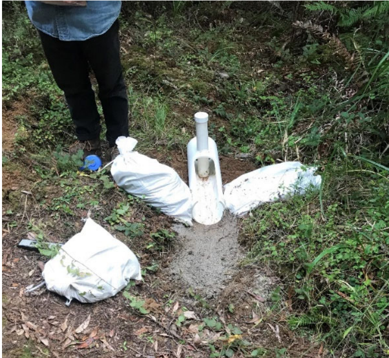
Figure 7. Homemade road flume placed in a road ditch of the South Fork of Caspar Creek. Concrete mortar and sand bags at the inlet ensured all ditch flow entered the flume. Some installations used clay or weathered sandstone to seal the flume inlet instead of concrete.
