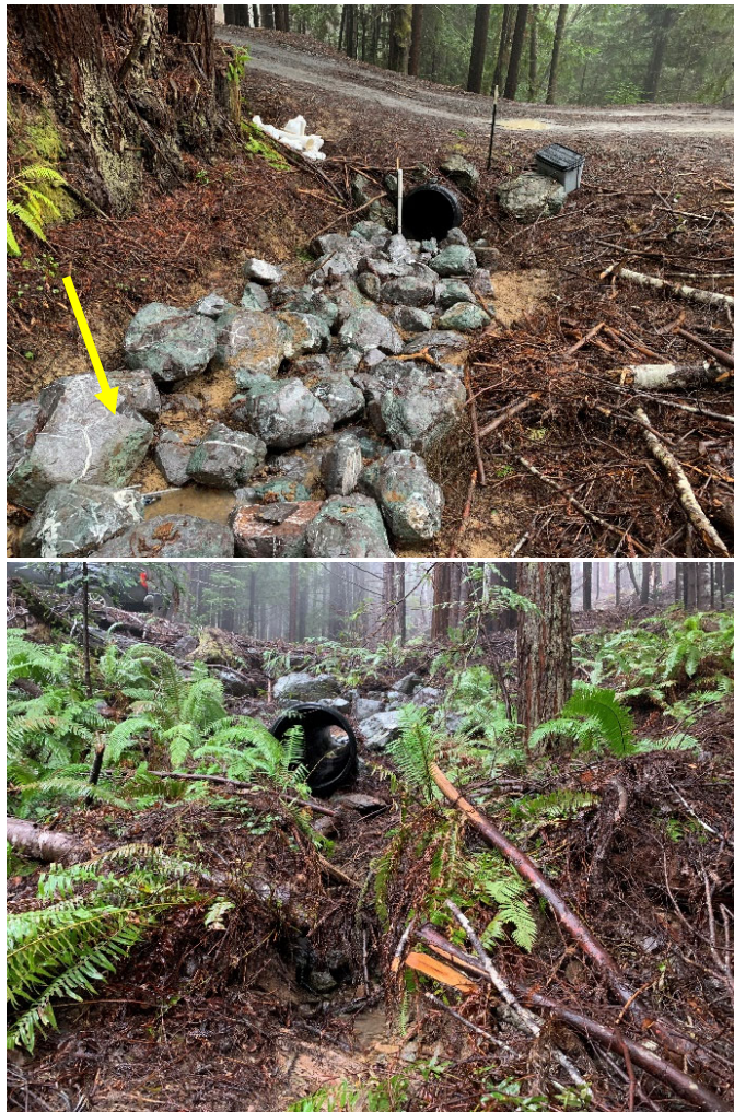
A B Figure 30. The inlet and outlet of the Class II watercourse. A) This plate shows the white PVC standpipe at the inlet of the culvert for stage measurement. At the lower left of plate A, amongst the rock is the turbidity probe. B) This plate shows the outlet of the crossing and demonstrates the steepness of the watercourse. The photographer is standing approximately 20 feet downstream and is 6.1 feet tall and looking up at the outlet.
